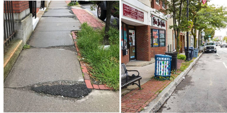
Example of poor sidewalk conditions along Cambridge St.
