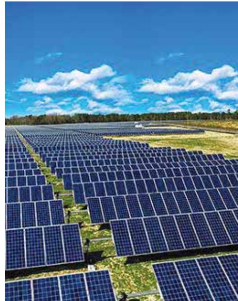
Figure 13. Example off-site PV installation
