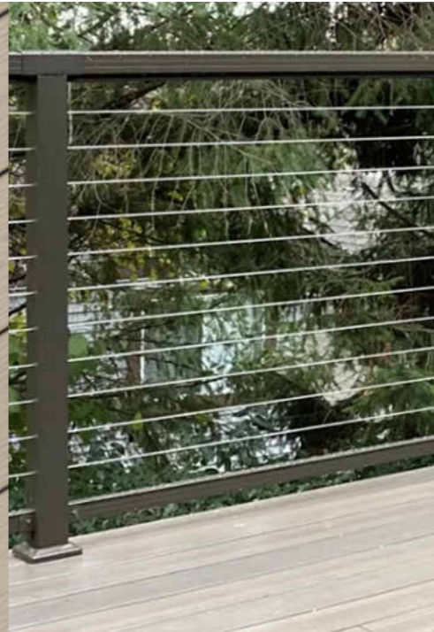
CABLE GUARD RAIL ELEVATED PORCHES & DECKS STAIRS & STAIR WELLS
