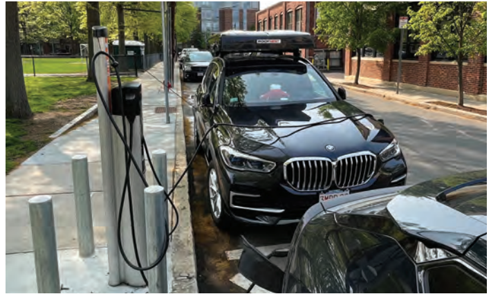
Electric Vehicle Charging Station at 29 Tudor Street.
