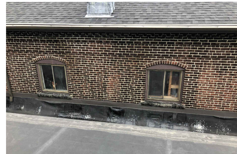
BARN LEFT SIDE - WINDOWS TO BE REPLACED
