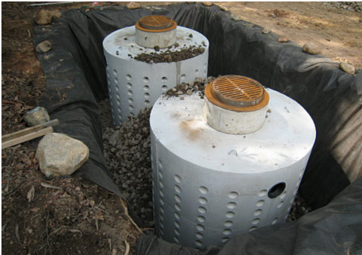
Leaching catch basin - Credit: Massachusetts Clean Water Toolkit: http://prj.geosyntec.com/npsmanual/leachingcatchbasin.aspx
