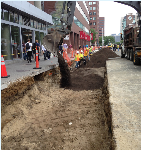
Main Street in Kendall Square showing the extent of sand based structural soil.
