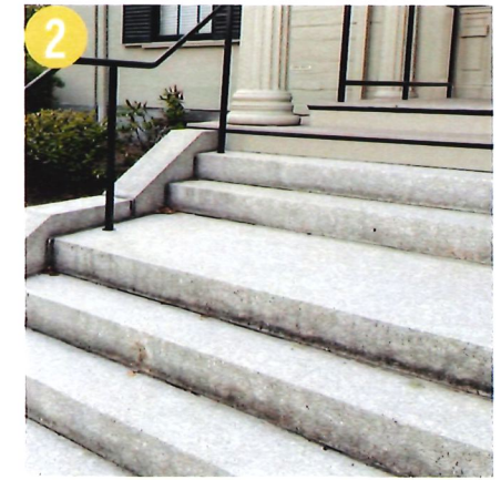
REPAIRED OR REPLACED GRANITE STAIRS
