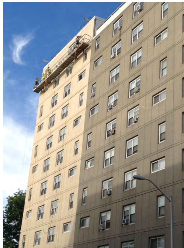
Putnam Square Apts.: 94 rental units preserved and now being rehabbed for senior and disabled tenants
