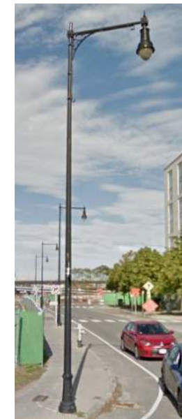
Light Pole - Street
