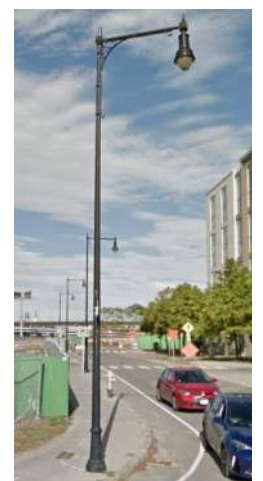
③ LP-S: Street Light Pole
