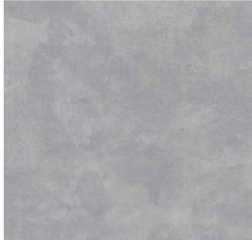
Polished concrete floor and ramp with a 0.43 coefficient for friction (required slip resistance)
