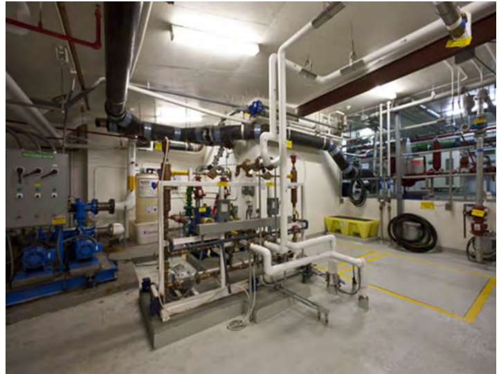
Figure 21. Image of blackwater treatment system in NYC project – Courtesy of Natural Systems Utilities
