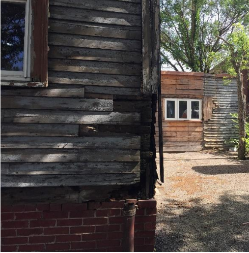
Southeast corner, showing rot of the corner post and sill. East side wing visible in background.
