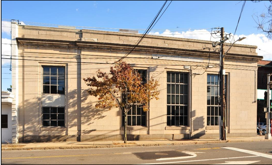
West elevation, November 2017. Cornice deterioration from water damage is evident.
