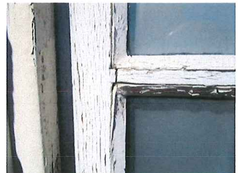
Group A & B- Sash cut for IGU. Paint, glaze, & wood in poor condition
