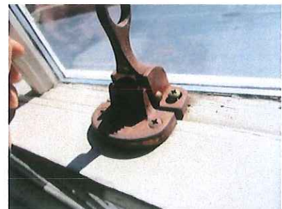
Hardware- Does not seem to be original, since they are designed for use on sash with a pole.
