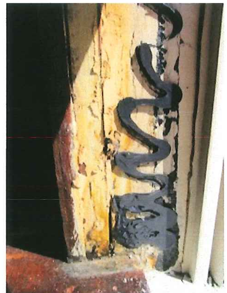
Group A & B- Lower sash with aluminum clad jamb and original paint behind
