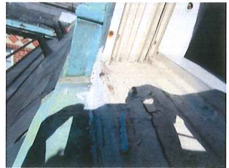
Group A- Copper clad exterior trim and sill requiring repair
