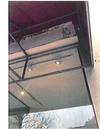
29 BRATTLE STREET, CAMBRIDGE, MA 02138 2019. 11.18 EXISTING LINTEL TO REMAIN AND TO BE COVERED WITH BLACK METAL BOX.
