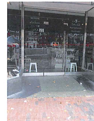
29 BRATTLE STREET, CAMBRIDGE, MA 02138 2019. 11.18 EXISTING ENTRY DOOR AND SIDELITE TO BE REMOVED. ALSO, RECESSED ENTRY FLOORING TO BE REMOVED.
