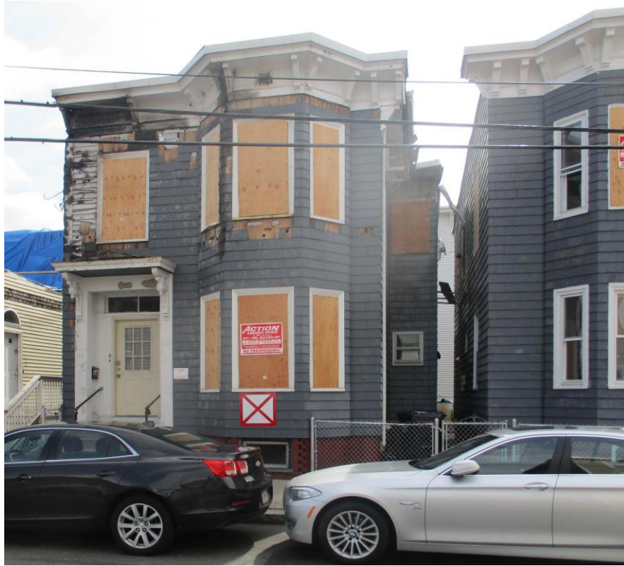
26 Berkshire Street post-fire
