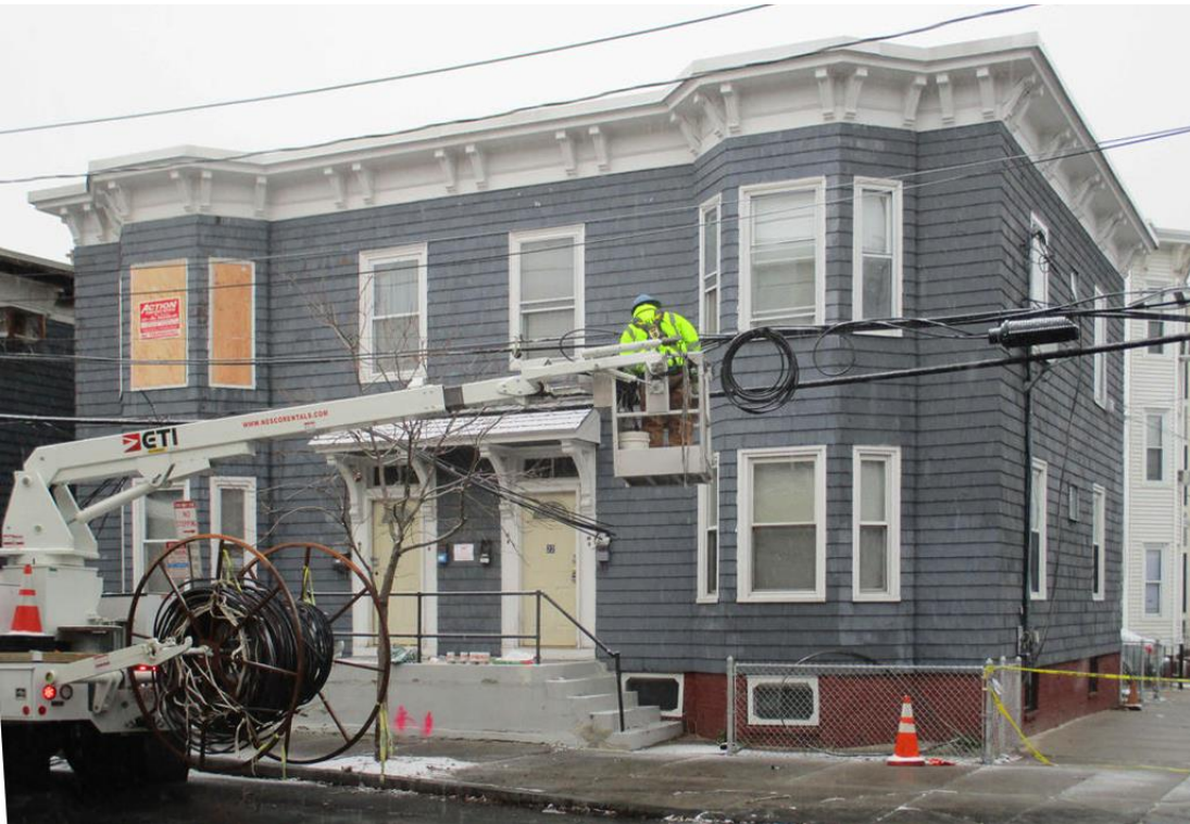
22-24 Berkshire Street post-fire.
