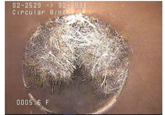
Root Intrusion in sewer pipe
