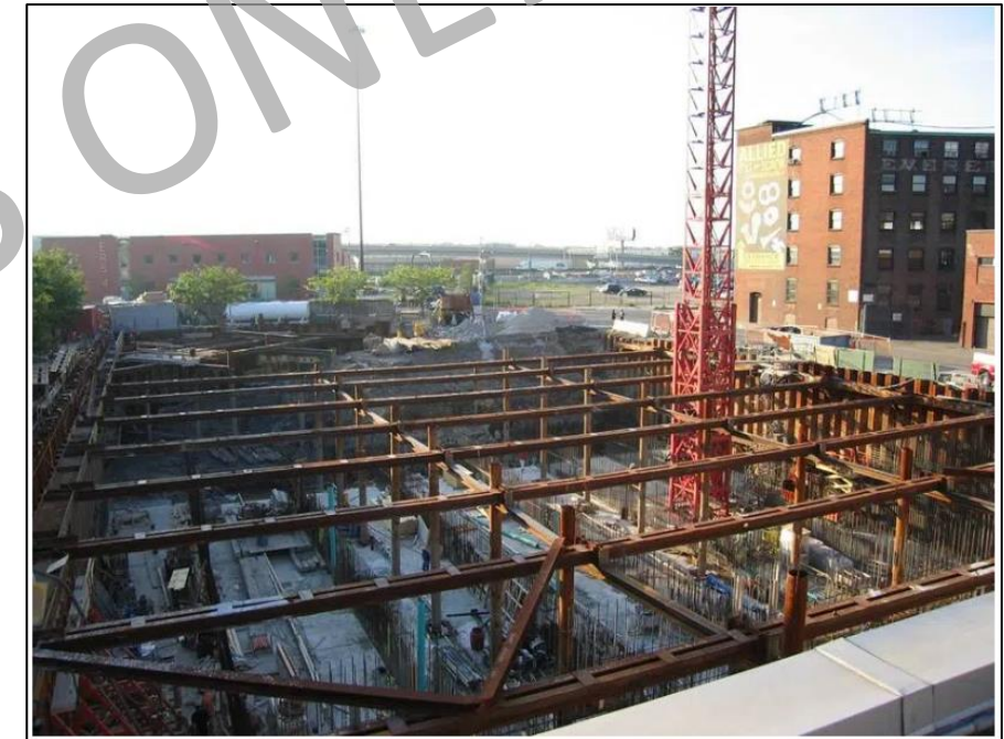
Union Park CSO Facility Storage Basins: Photo Credit: Simpson Gumpertz & Heger (SGH)
