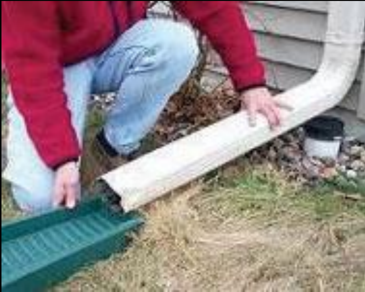
Downspouts disconnected. Elbow capped.
