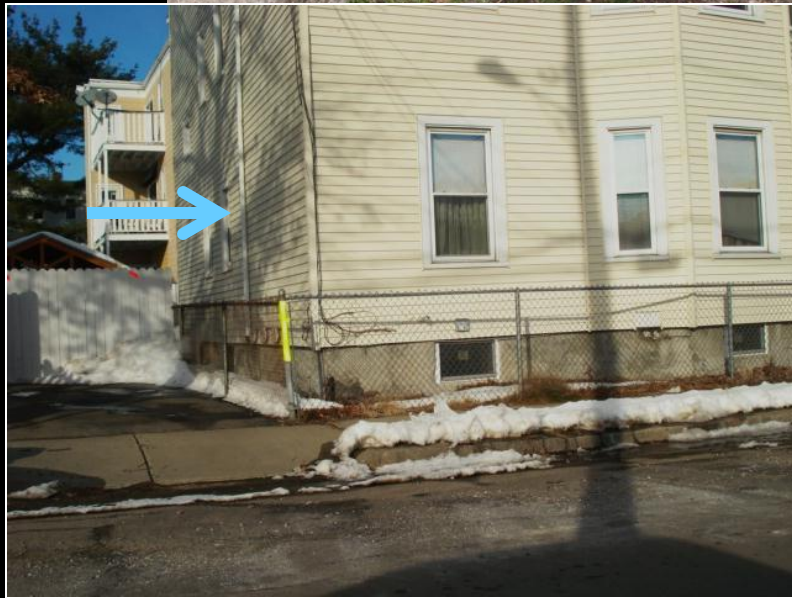
Before: Downspout disappeared into foundation; connected to sewer
