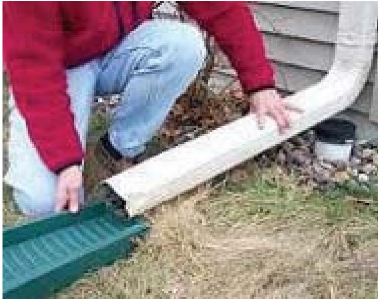
Downspouts disconnected. Elbow capped.
