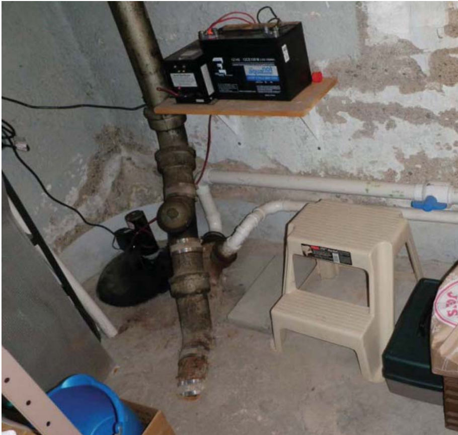
Before: Roof Leaders and Sump Discharge Tied into Sewer
