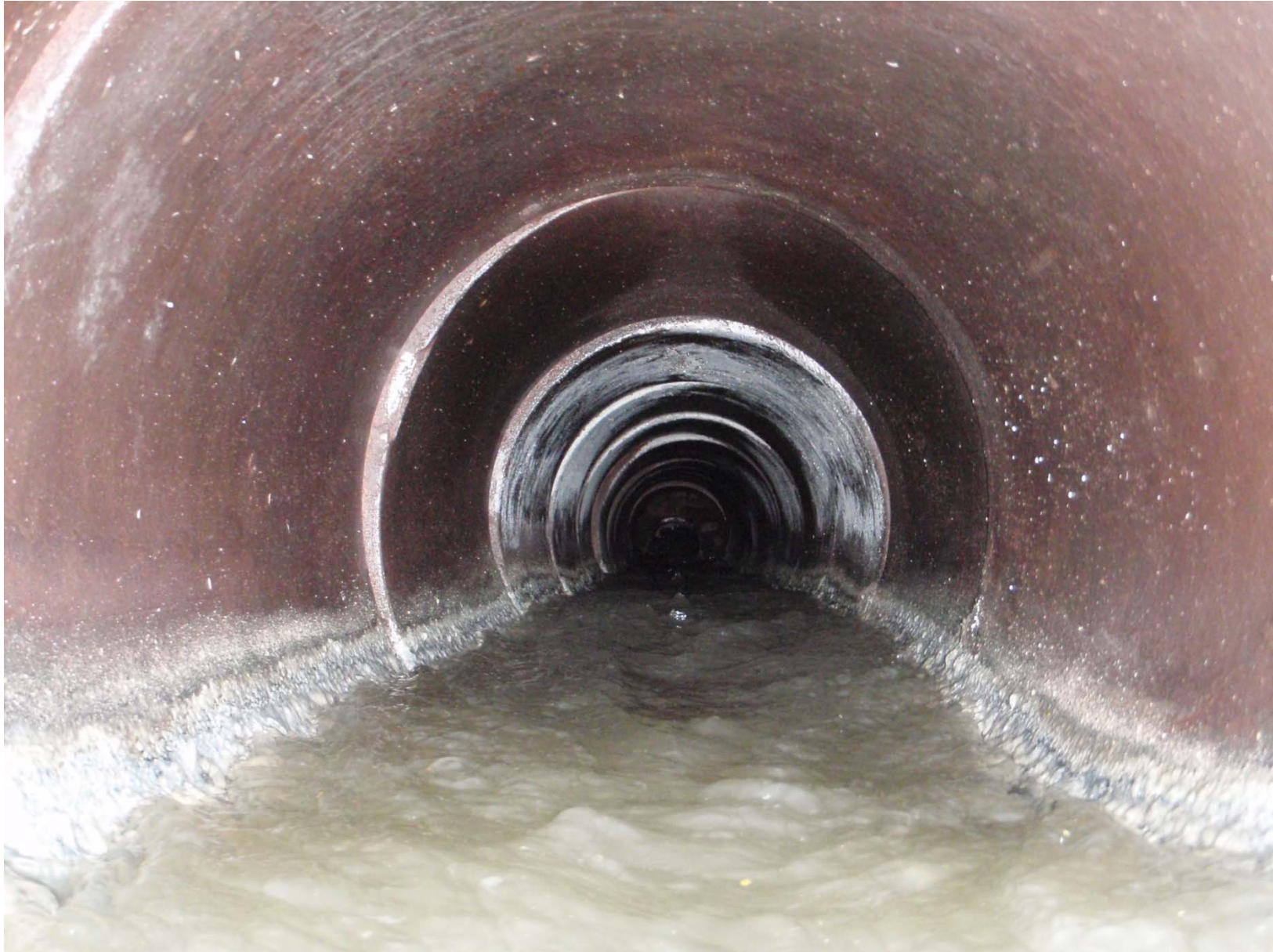
CAM 401B underflow – Looking upstream from junction with 66" MWRA Sewer into 18" pipe toward 401B regulator. 10" diameter masonry orifice visible at upstream end of pipe
