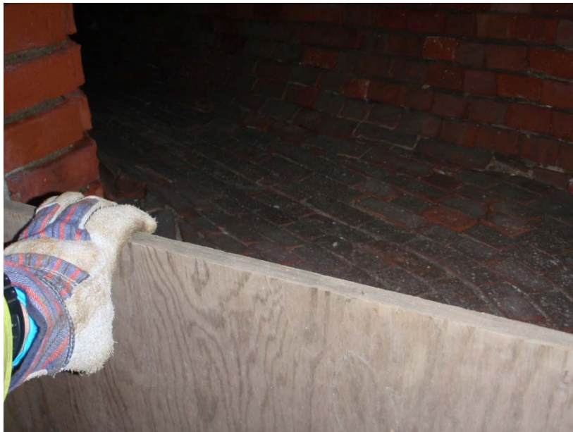
CAM 002A Overflow with weir
