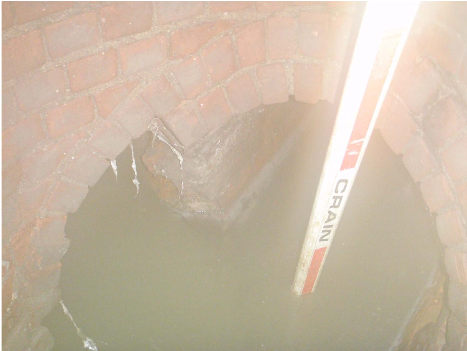
CAM 401B – Mass Ave & Magoun St sewer manhole. Orifice created due to break in by Mass Ave sewer at left. Mass Ave sewer reduces from 30"W x 41"H to 22"W x 30"H at manhole entrance
