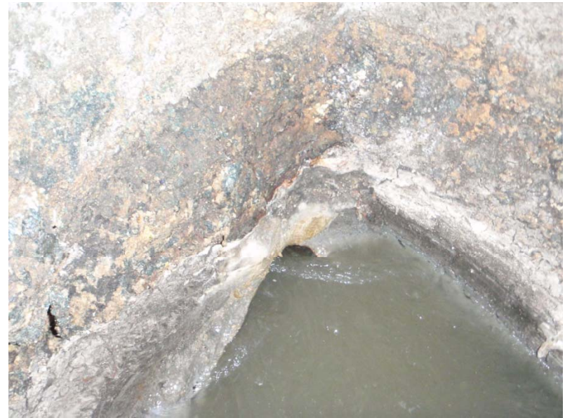
CAM 401B - 10" Masonry orifice underflow
