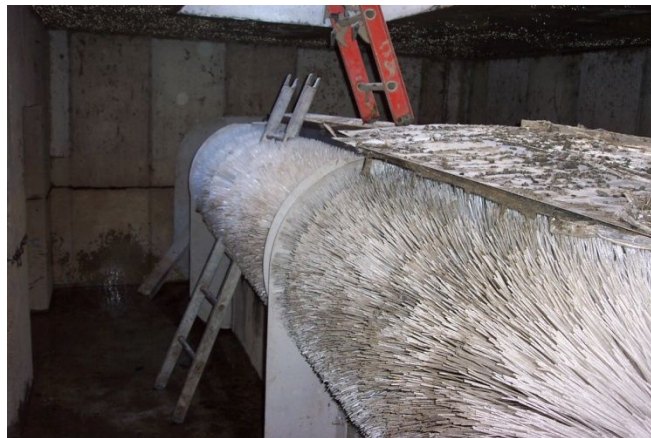
Figure 5 – Floatables Control Brush Screen within CAM 401A Regulator
