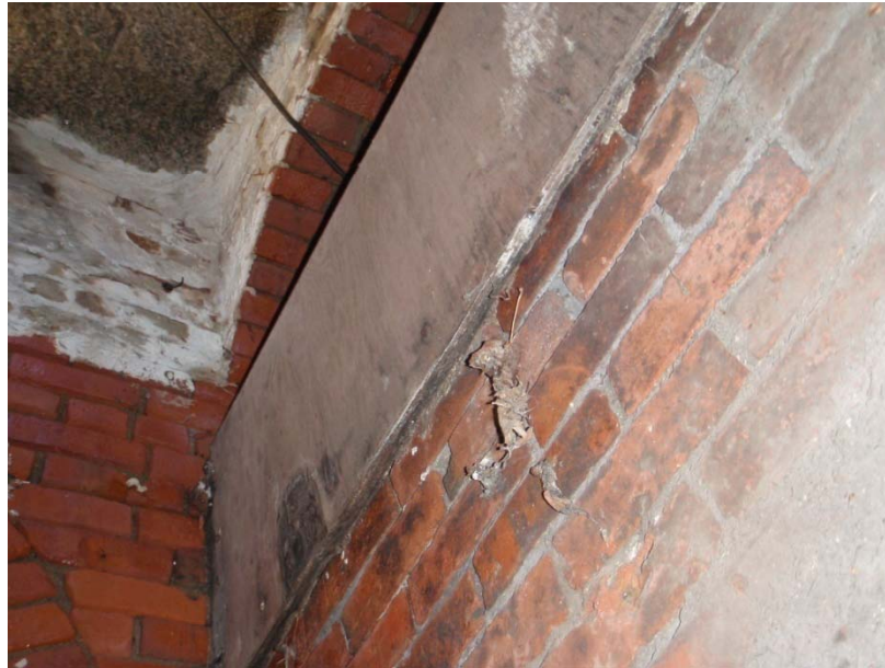
CAM 002A Overflow (with partial weir blockage)
