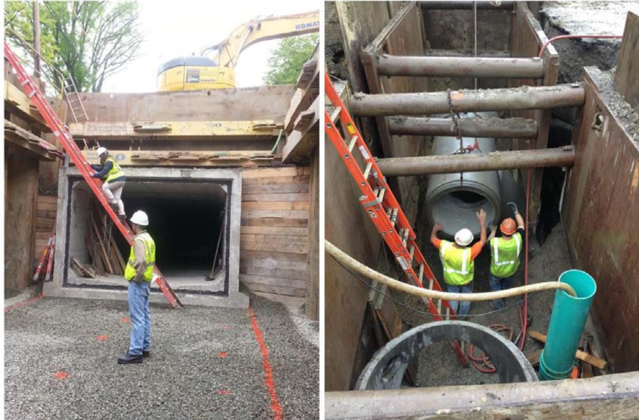
(L): Construction of a 160,000 gallon storm water holding tank on Hovey Street to reduce flooding in the Agassiz neighborhood. (R): Installation of 36" drain pipe, Western Avenue.
