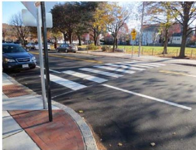
(L): Installation of new curbing associated with sidewalk reconstruction at the corner of Bryant and Scott Streets
