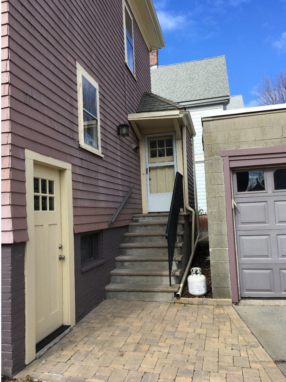
SOUTH FAÇADE OF 103 BELMONT, SHOWING FIRST FLOOR WINDOW TO BE REMOVED. NEW, SMALLER WINDOW IS PROPOSED TO BE INSTALLED SLIGHTING LEFT OF EXISTING WINDOW.
