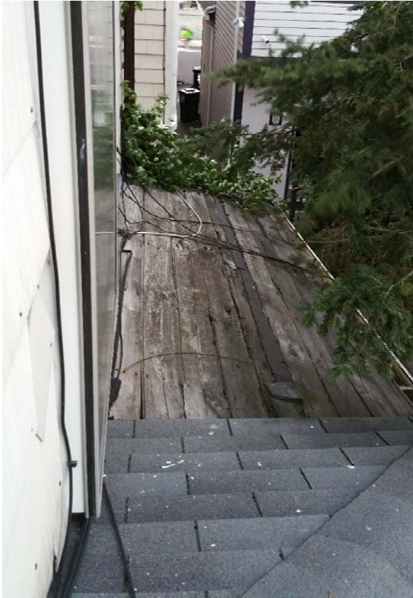
Existing rear porch as seen from second floor rear window (looking east)
