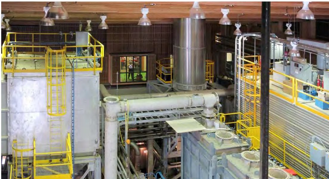
UBC Biomass Plant (Integral Group)
