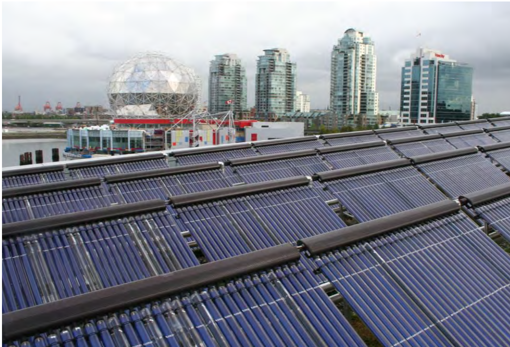
Vancouver Creekside Community Centre Solar Thermal Installation (Integral Group)
