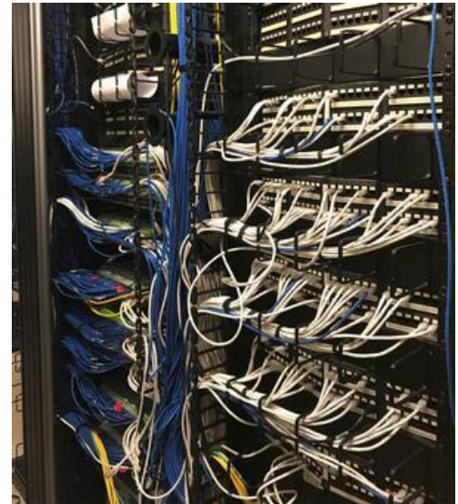
Public Safety Server Room.
