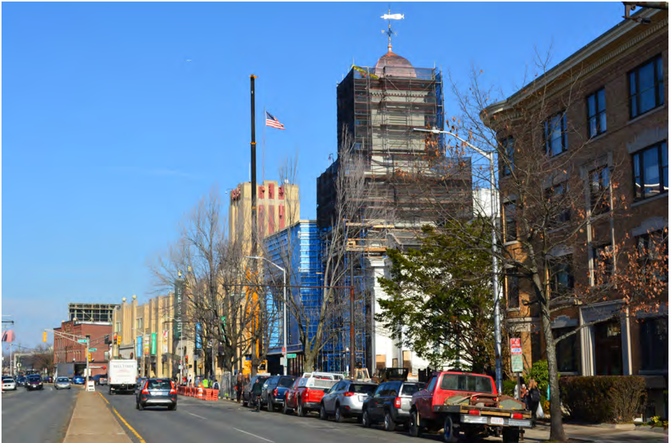
THE LUNDER ARTS CENTER NEARING COMPLETION, DECEMBER 1 2014, THE RESTORED COPPER CUPOLA VISIBLE BEHIND SCAFFOLDING.
