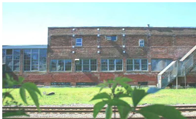
7 Rear Side of Existing Building Showing Areas of Repaired Facade Failure
