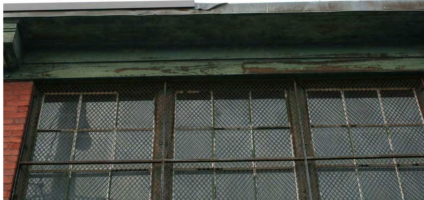
Roof eave requires significant repair. Windows and trim need replacement.
