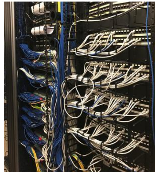
Public Safety Server Room.
