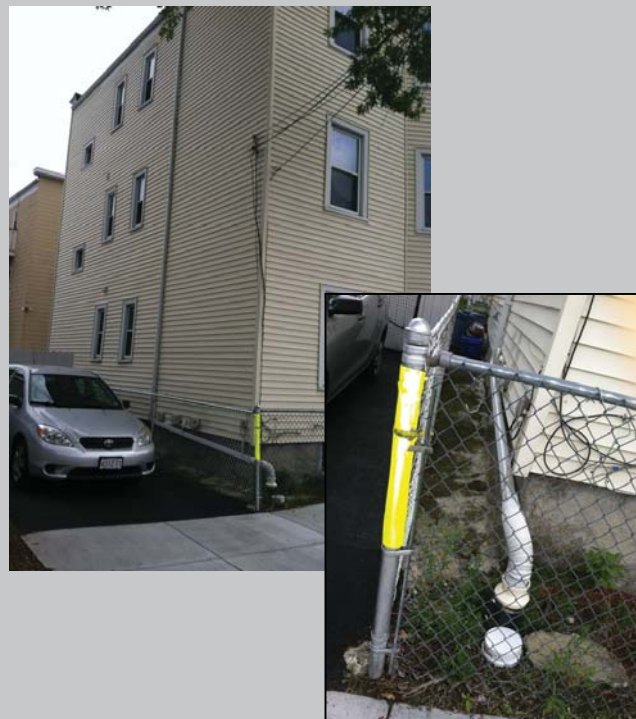
AFTER: Downspout reconnected to new drain lateral with cleanout access. Sidewalk and driveway restored.
