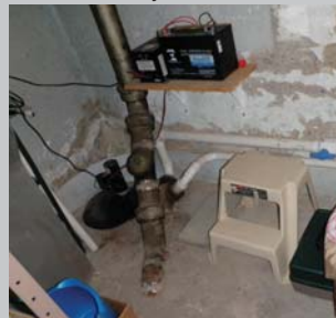
B. Sump pumps hard-piped to sanitary sewer service
