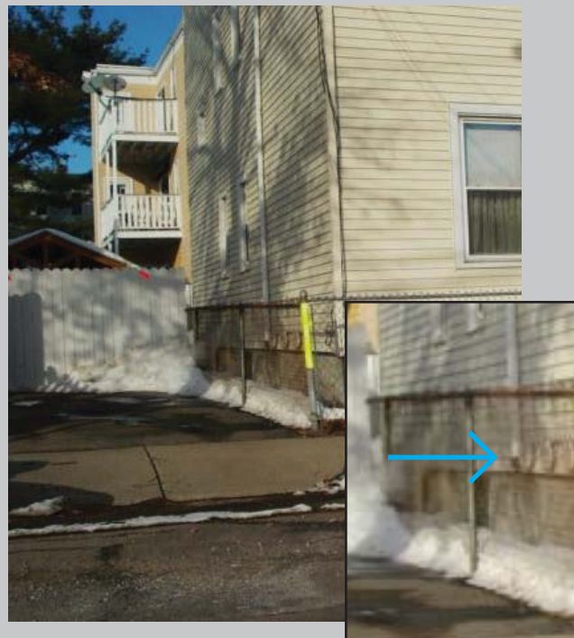
BEFORE: Downspout disappeared into foundation; connected to sewer
