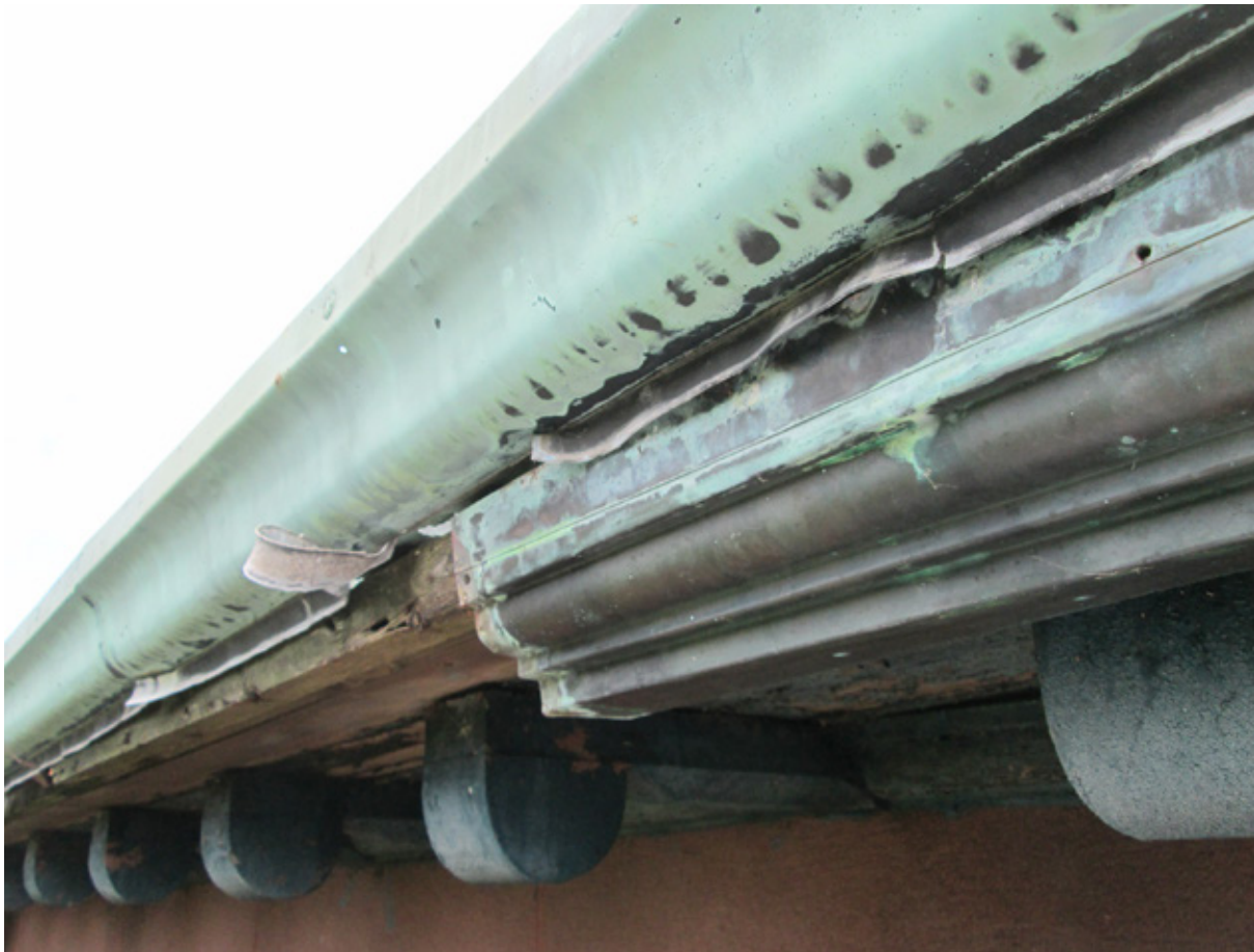
Damaged and missing copper gutter and decorative cornice flashing.
