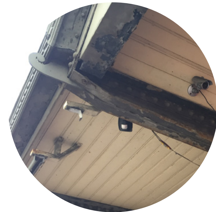
clean structural members for removal of rust and paint, to be repainted in the historic color
