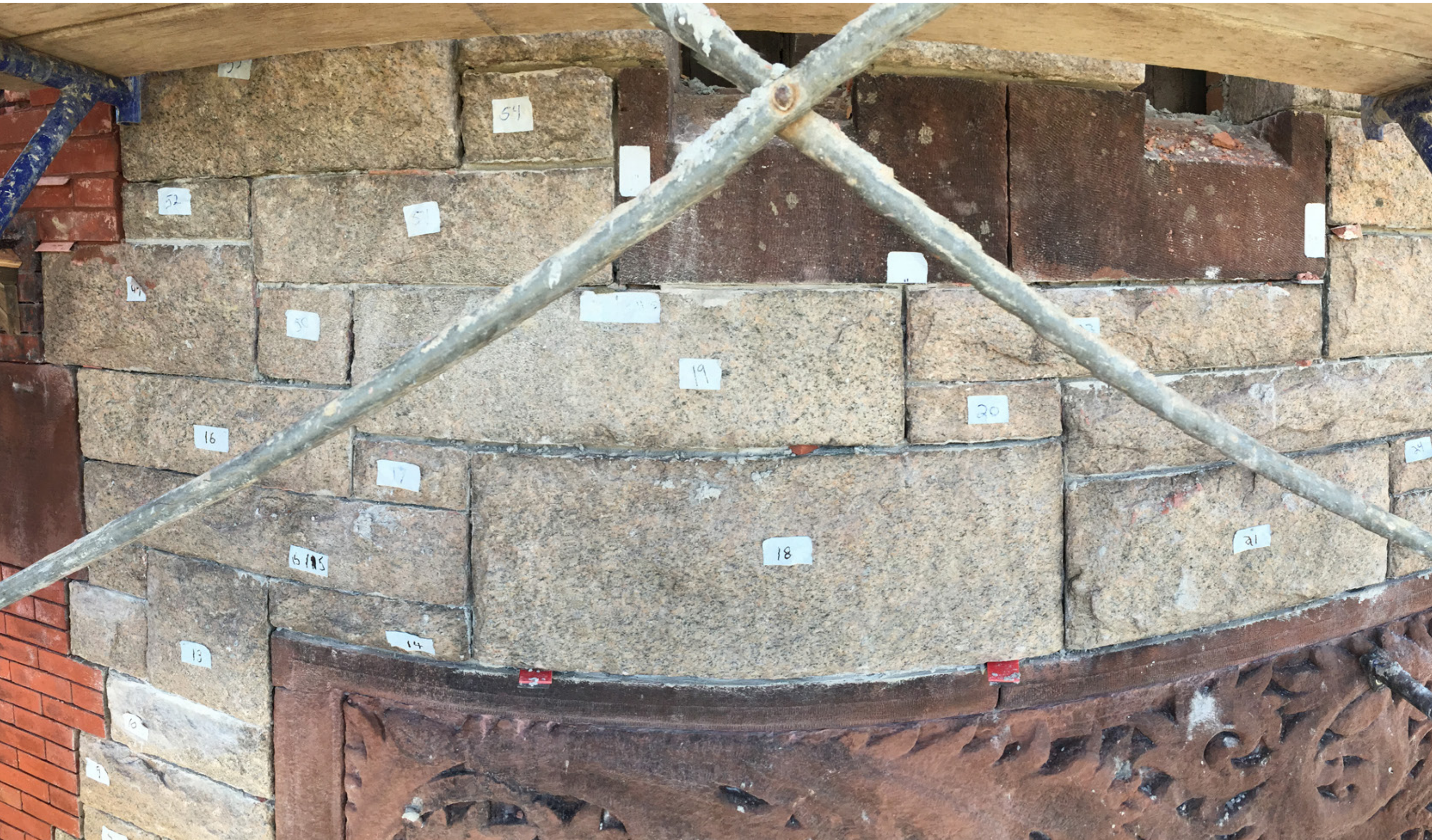
Due to extensive water damage and separation of the north wall from freeze thaw cycles, a large portion of the north facade needed to be rebuilt. The random ashlar granite blocks & brownstone details were tagged with identifying number's for careful removal. The brick backup wall was rebuilt and the random ashlar pattern was relaid in it's original pattern.
