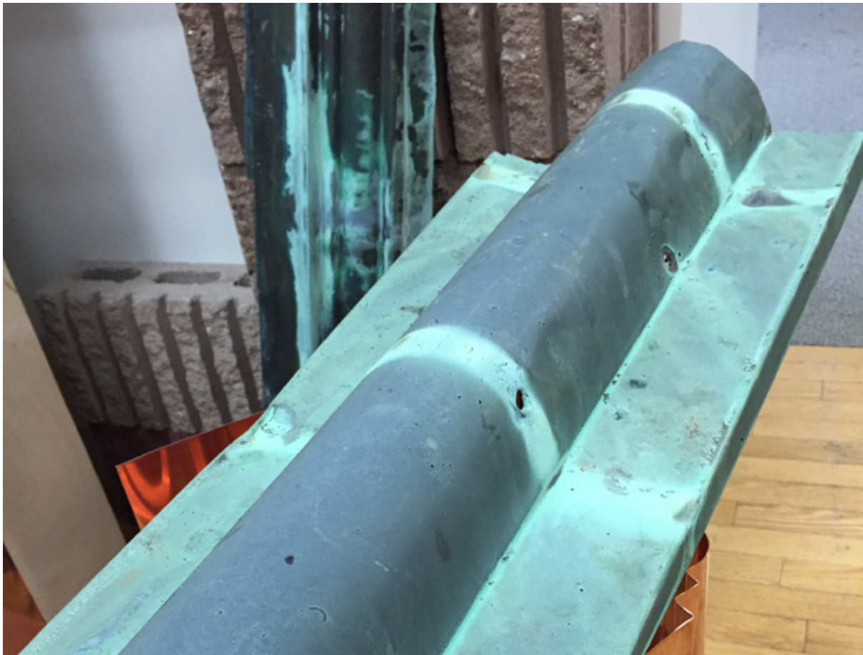
Original copper hip roof ridge detail with missing brackets.
