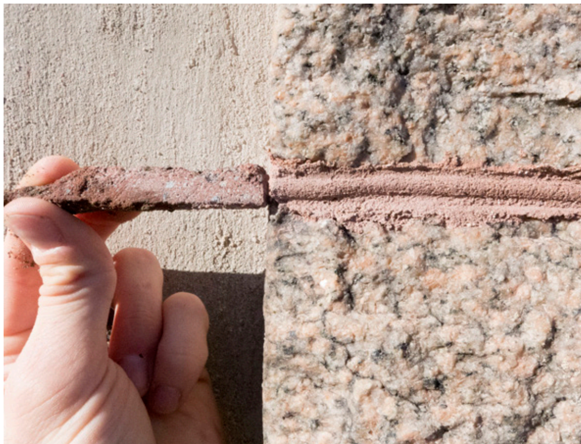
Comparison of original mortar to proposed mortar color and tooling. Masonry cleaning (above).
