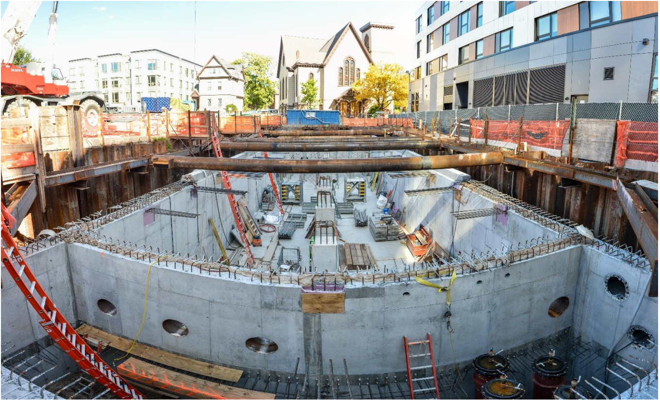
Construction on an underground tank in The Port that captured almost 3.5 million gallons of stormwater water during summer 2021
