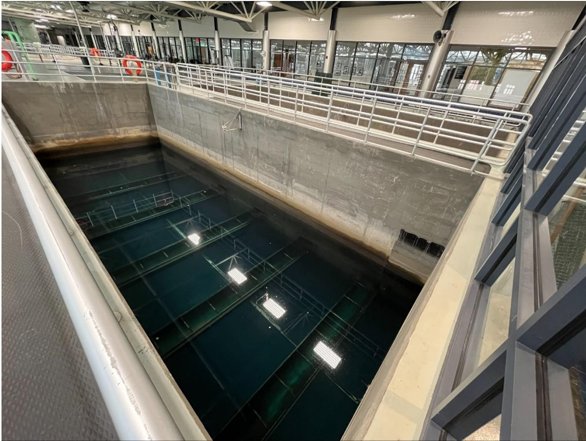
One of the water filters with newly replaced granular activated carbon media
