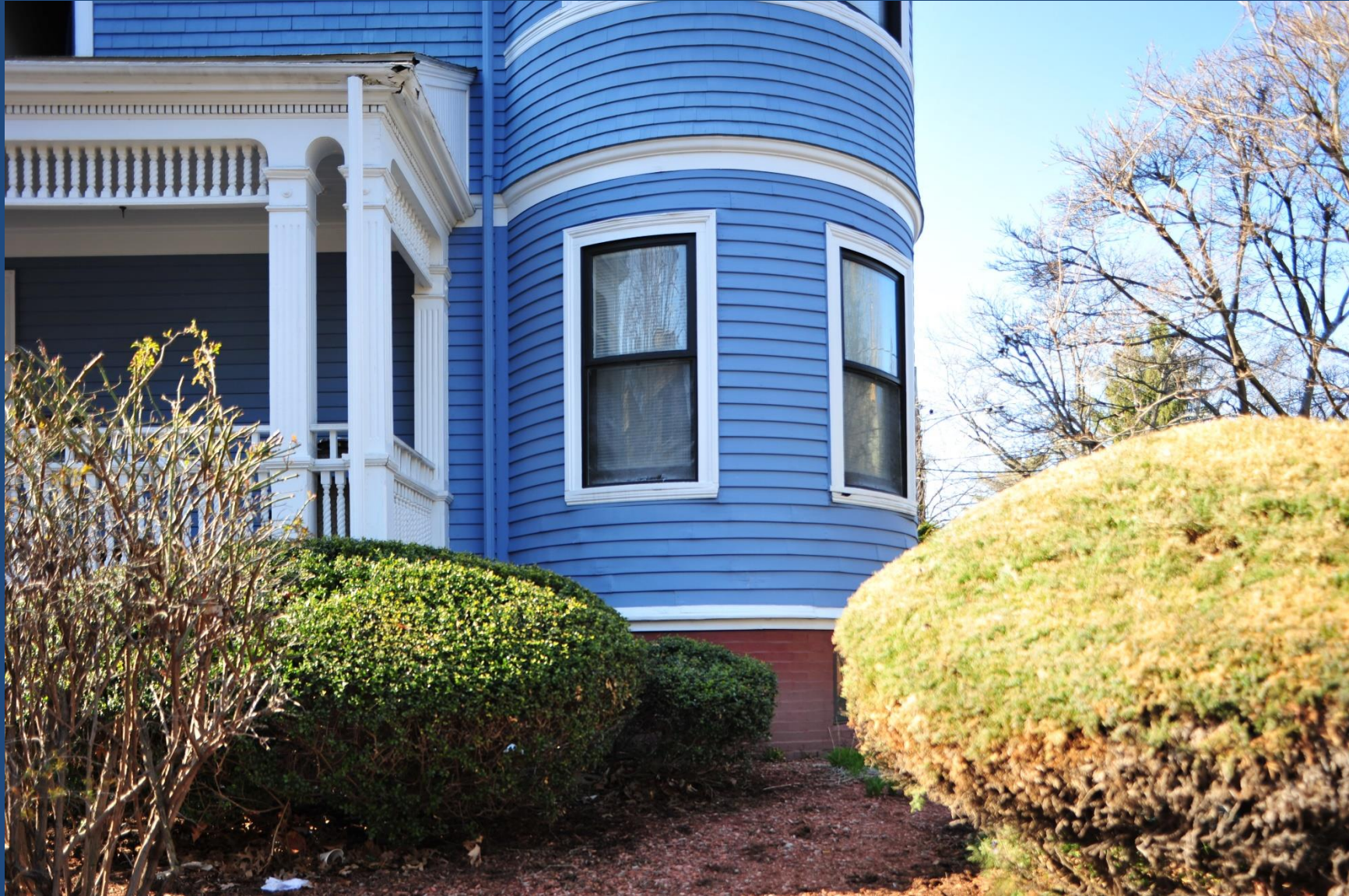
PG 20-05, 71 Hammond Street, by Cambridge Housing Authority. $50,000 for siding and porch repairs
