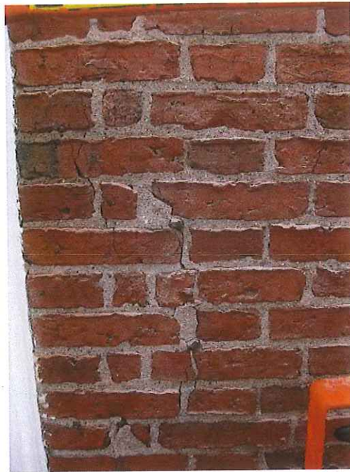
Cracked brick and "hard" cement based mortar
