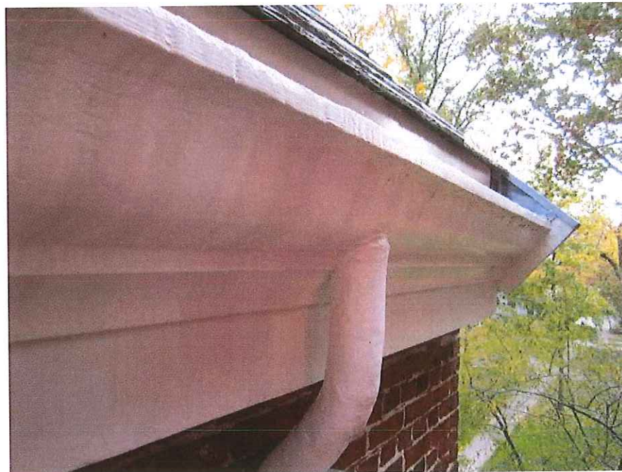
Existing painted wood gutter and gooseneck
