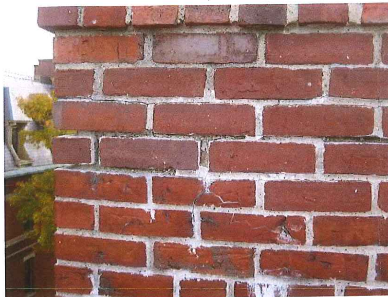
Deteriorated mortar joints at chimneys
