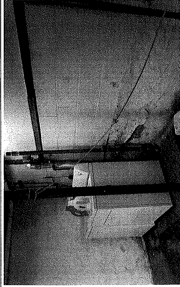
View inside of lower level. New CMU constructed on top of rubble foundation wall.
