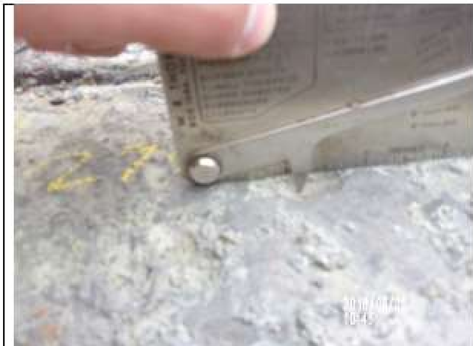
Pipe close-up, 270 mil gouge
