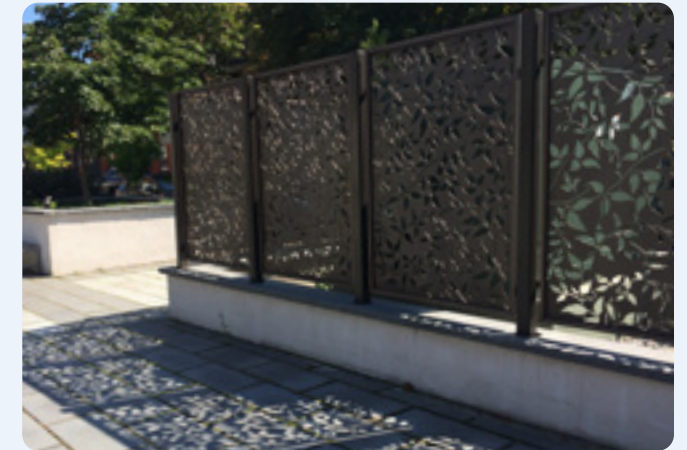
FIG. 25 Transformer and switchgear are thoughtfully screened and integrated into the landscape design to minimize visual impacts
