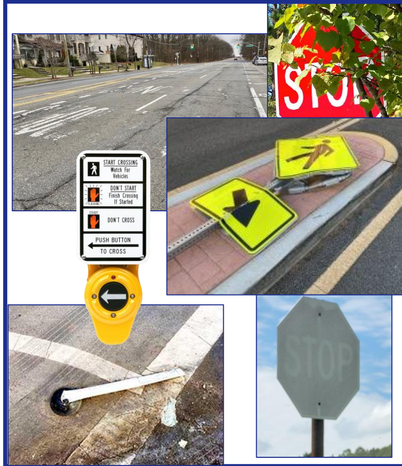
Maintenance of Safety and Accessibility Devices
