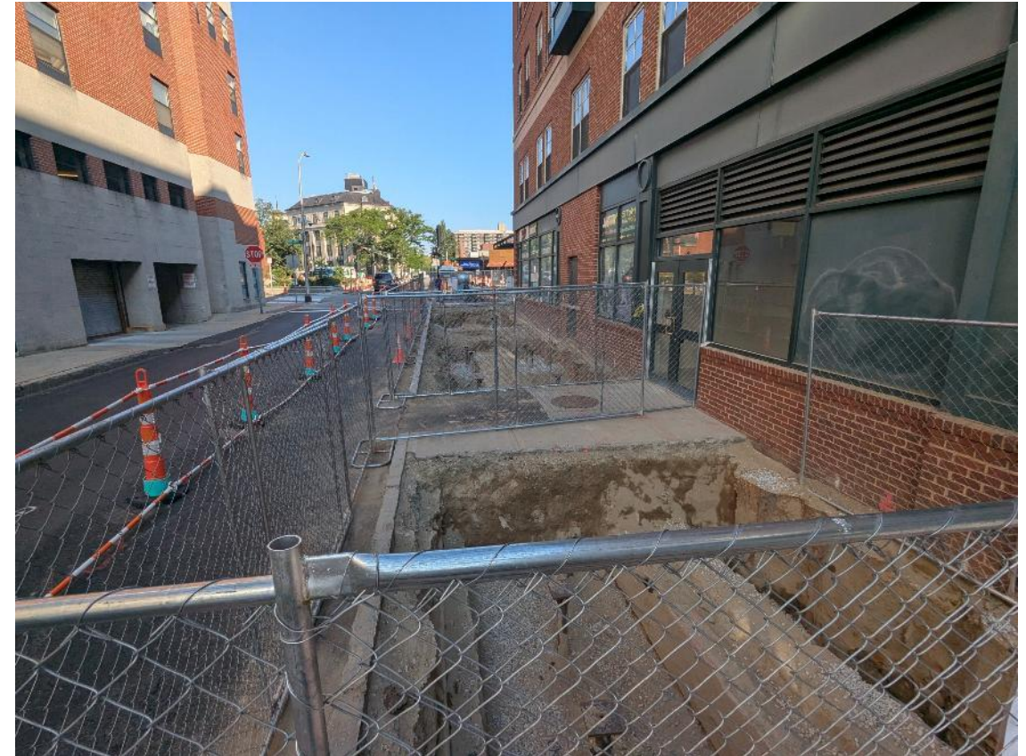
Image: Excavated sidewalk on Green Street. Underground utility conduit and supports for future foundations visible.
