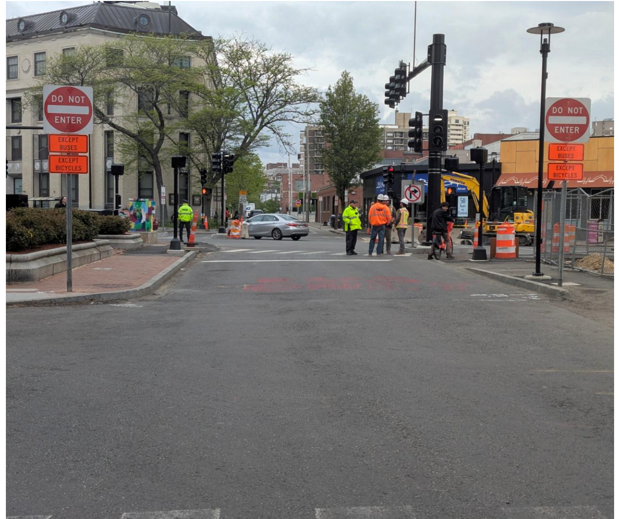
Image: New traffic signal at Green Street and River Street and new traffic signage restricting Green Street to buses and bikes only.
