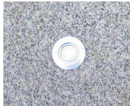
Uplight - main entry sign
