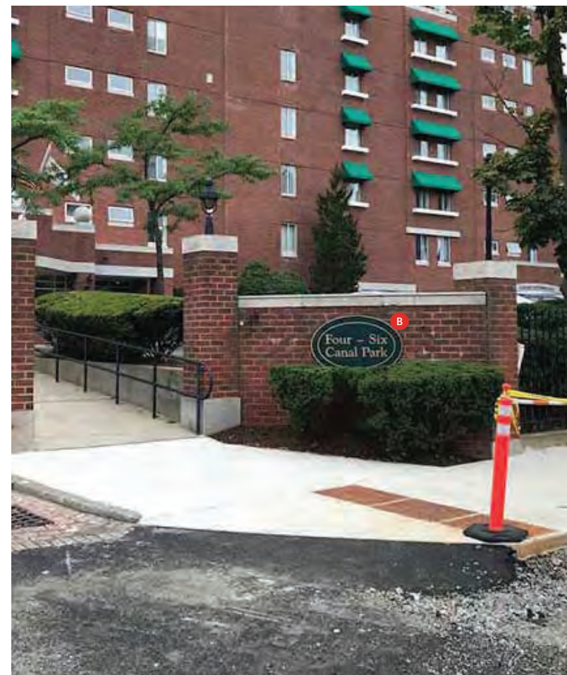
B Entry sign on wall at curb cut
