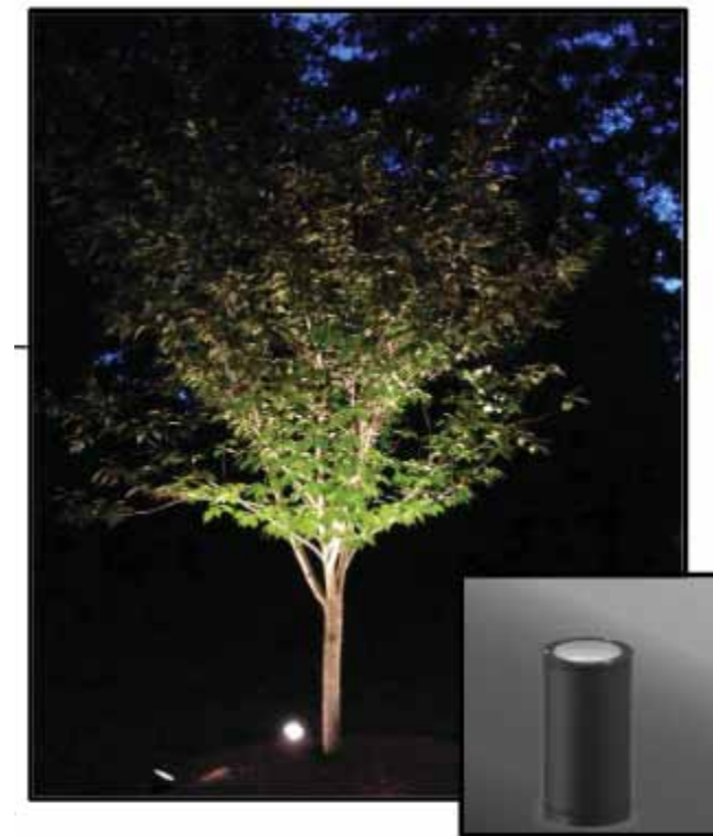
Dimmable, 3000K above-grade tree uplighting to be controlled automatically via programmable astronomic time clock
