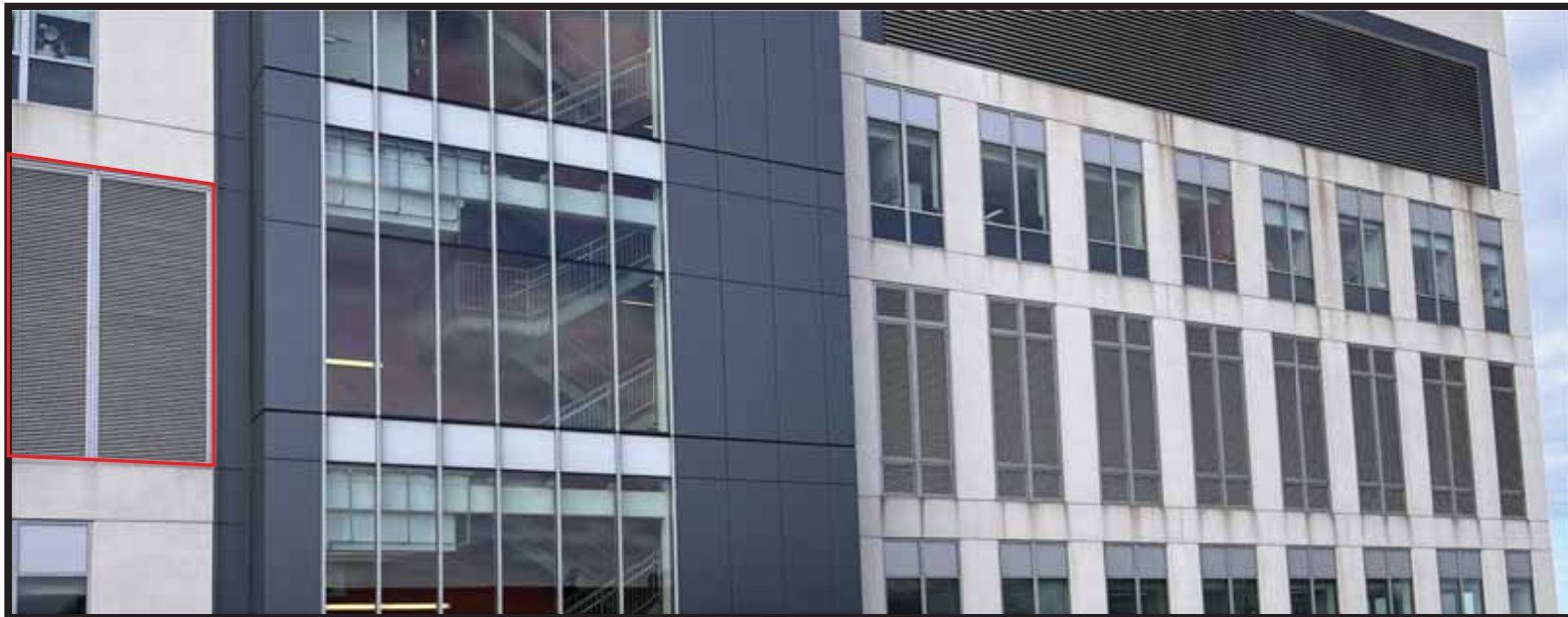
EXHIBIT E-3: REMAINING FACADE. RED BOX IS EXTENT OF BROAD PROPOSED WORK
