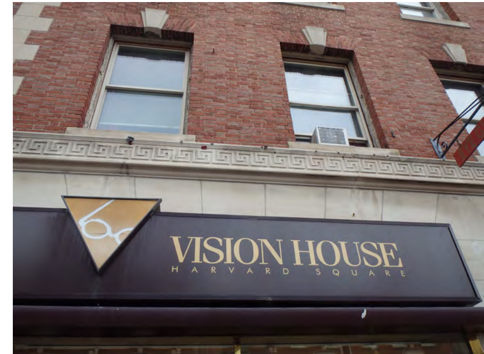
FERROUS ANCHORS, CONDUITS, AND ATTACHMENTS TO BE REMOVED AND RESULTING HOLES PATCHED
