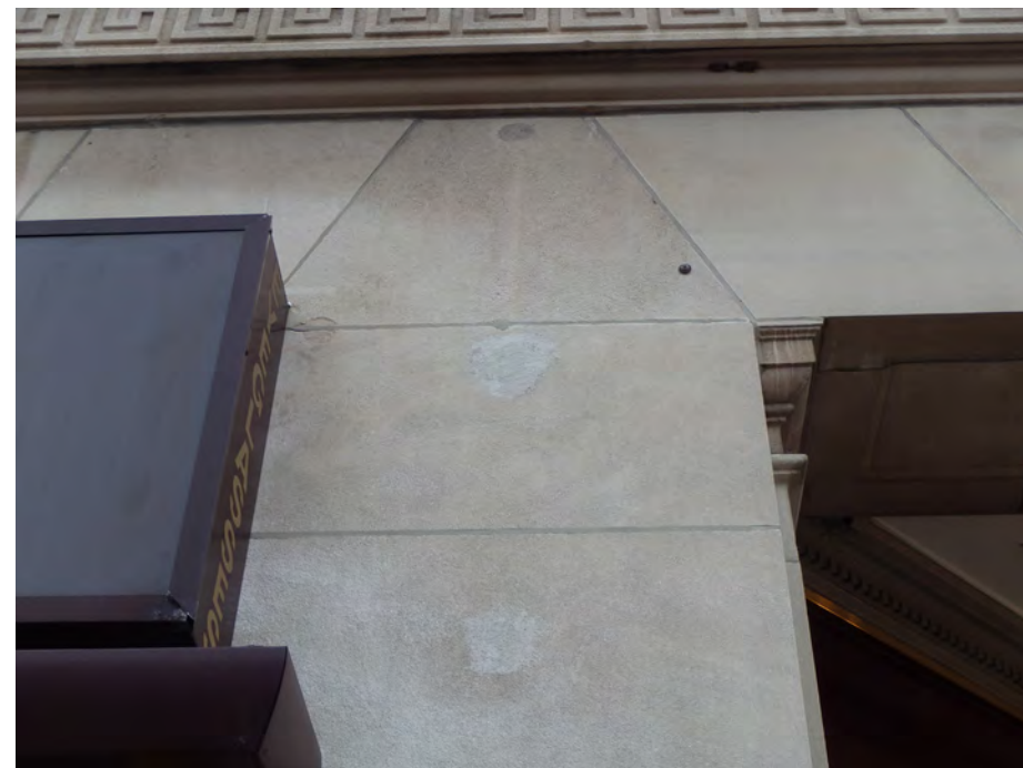
PREVIOUS LIMESTONE PATCHES TO BE REMOVED AND NEW PATCHES INSTALLED TO MATCH SURROUNDING STONE
