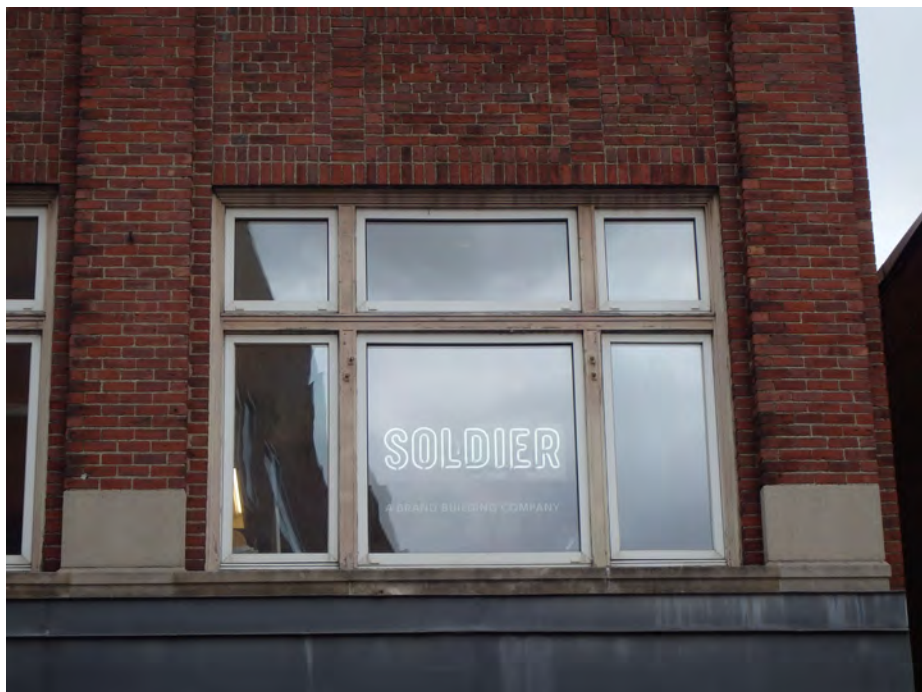
WOOD WINDOW FRAMES TO BE RESTORED. WOOD WINDOW SASH TO BE REPLACED TO MATCH ORIGINAL PROFILES AND CONFIGURATION.
