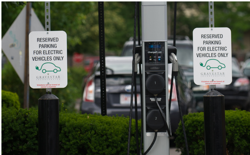
Electric vehicle charging stations in a Cambridge parking lot.
