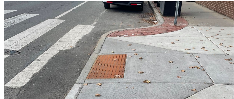
Image: Recently reconstructed curb ramp at Cambridge Street and Cardinal Medeiros Avenue
