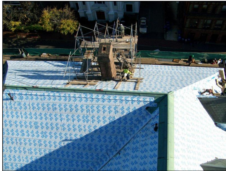
Slate roof replacement at City Hall to preserve it as a historical structure, FY13.
