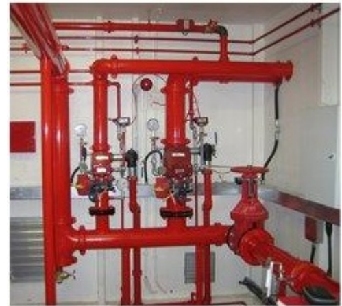
The duties of the Cambridge Fire Prevention Bureau include inspecting fire detection and alarm systems.
