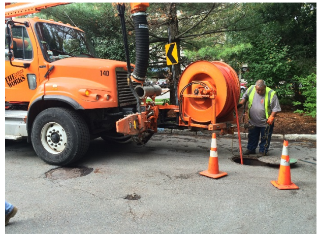
Public Works maintains 244 miles of sewer and stormwater pipelines.
