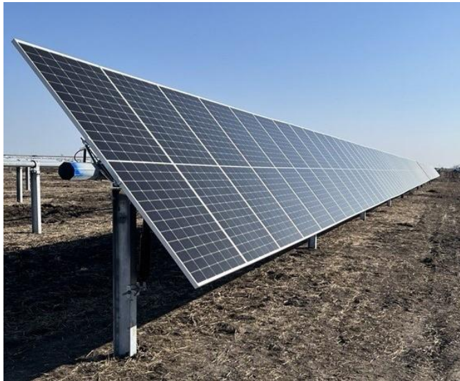
City-supported solar panels being installed at the Prairie Solar project in Illinois
