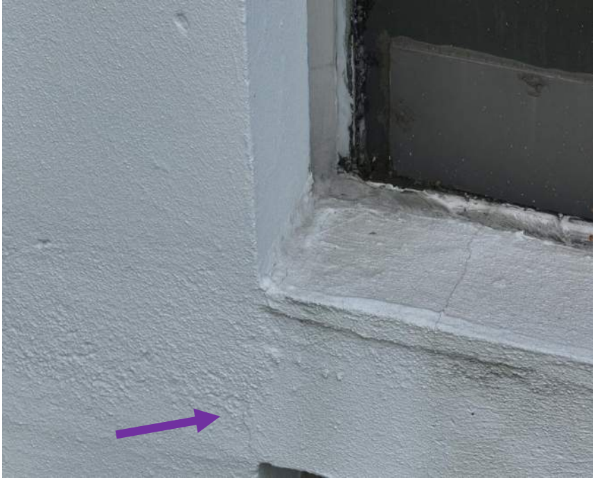
18 June 2024 Drone Survey, IMG#10-098 (cracks cannot be discerned from other photos, i.e. IMG#10-097)
